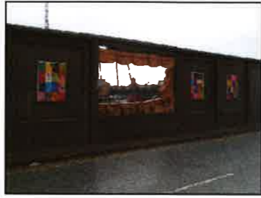
Photo 102 Hole in the wall of Hythe Quay.
